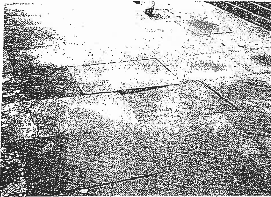
PAVING SLAB TRIP IN FOOTWAY
